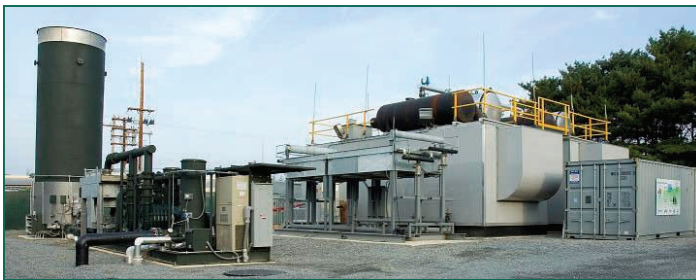
Landfill Gas-to-Energy Plant located in Conestoga, PA Manor Township, Lancaster County
