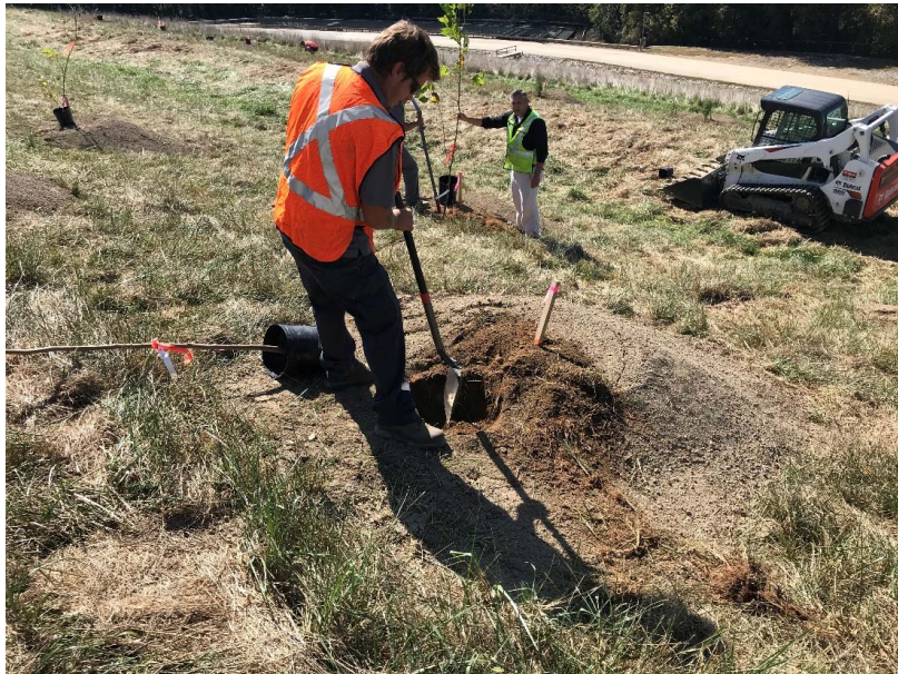
Photo 2 – Tomlinson Bomberger performing planting of the Phase 1 trees. All trees were planted with hand tools and monitored for planting depth by ARM.
